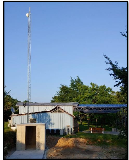
The Power-Comm Vault and Communications Tower next to the MobbyMac Carriage House Photo by G. Myers 6.23.21
