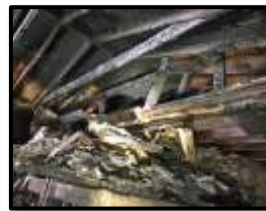
Interior damage Photo by: Servpro, NWA 4.4.20
